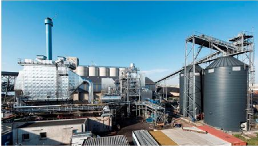
Above: the new biomass boiler
